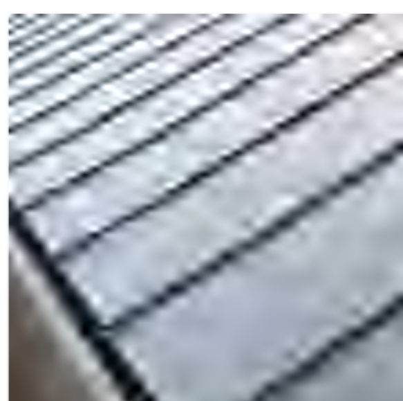
05 - Zinc (or equiv) standing seam roof cladding with integral concealed gutter in Dark Grey
