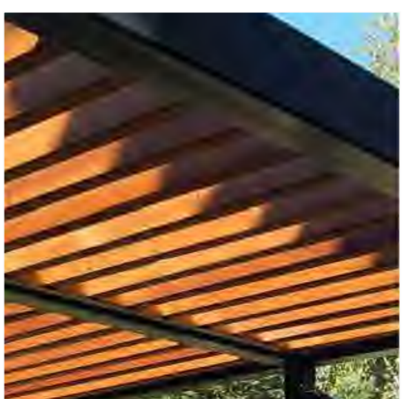
07 - vertical timber slat canopy set into dark grey metal frame to match glazing system
